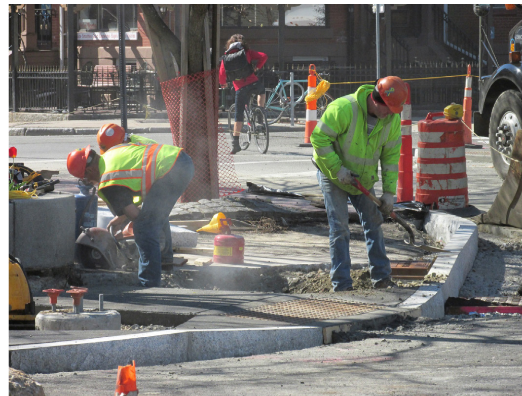
Workers reconstruct sidewalks along Western Avenue. The City implemented this street redesign to replace deteriorated sewer, drain, and water infrastructure; increase pedestrian and bicycle safety and comfort; improve bus amenities; and improve sidewalk management through additional green space and pervious pavement.
