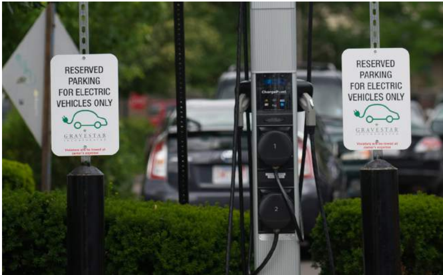
Electric vehicle charging stations in a Cambridge parking lot.
